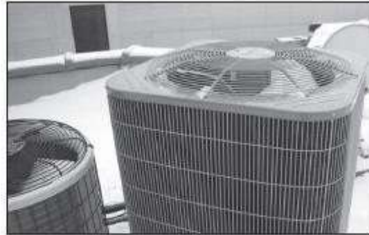
Air conditioning systems
